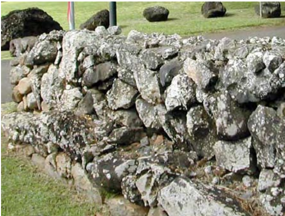
Example of dry stack wall which will be used in public and open spaces
