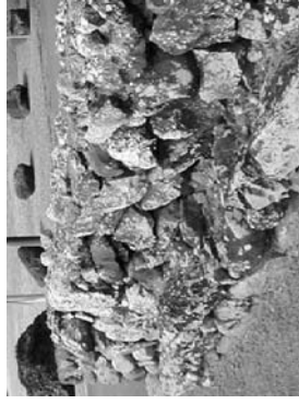
Example of dry stack wall which will be used in public and open spaces
